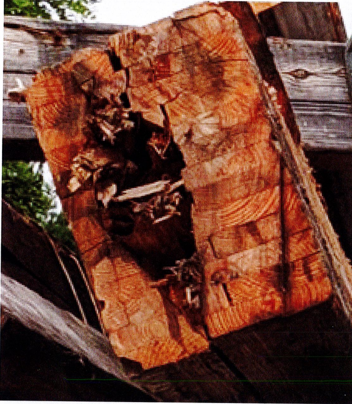
Sample - Laminated Wood Structure Rot
