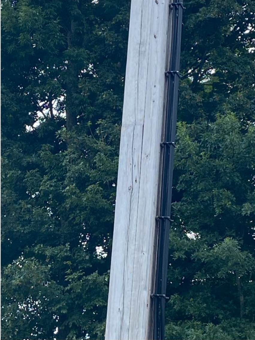
structure 8011 cracking from wood rot
