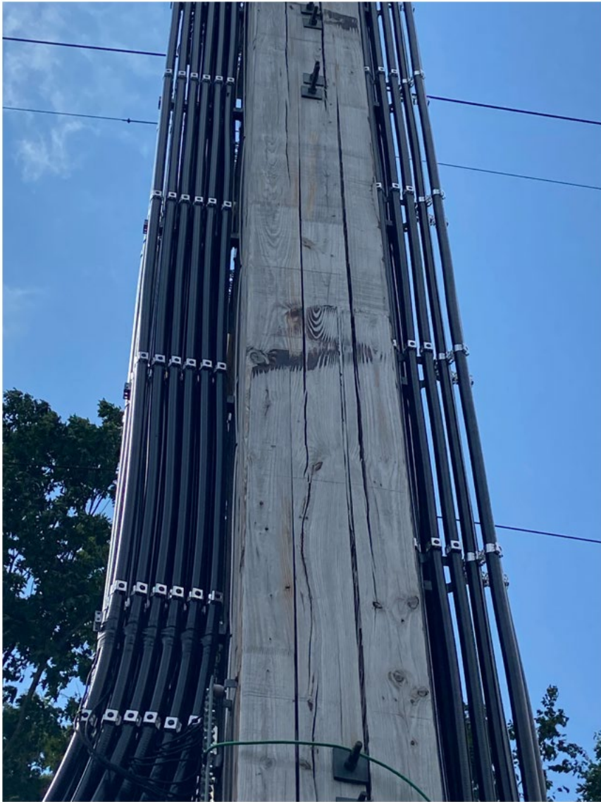
Structure 8011 cracking from wood rot
