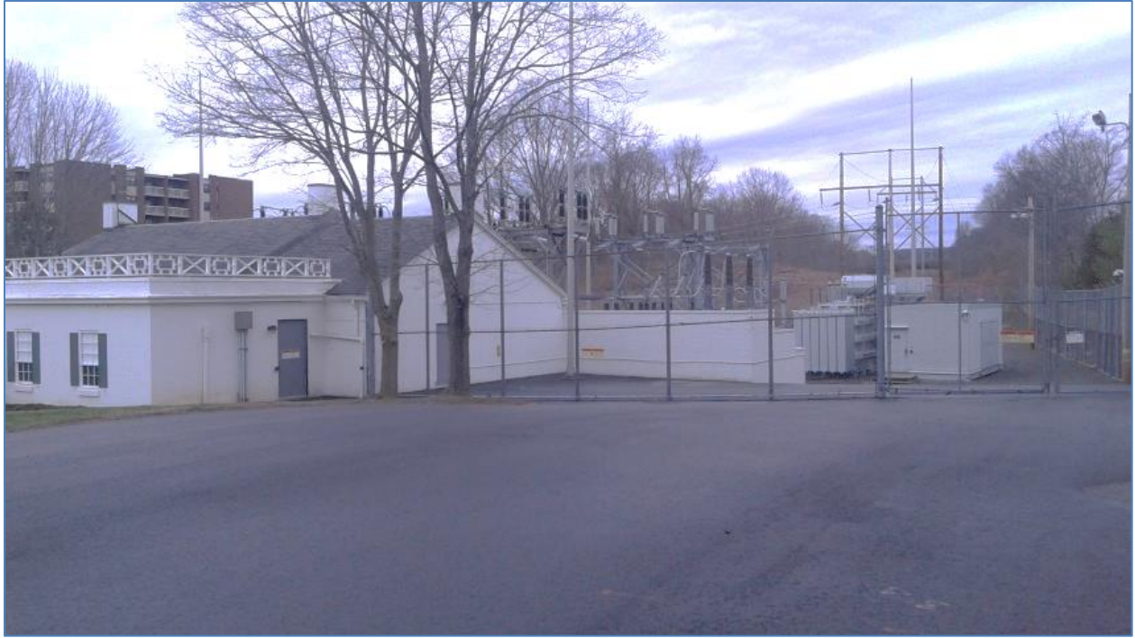
Photo 1. Overview photo of the existing Mix Avenue Substation facing southwest.
