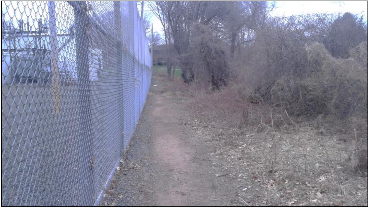
Photo 12. Overview photo of the area to the south of the Mix Avenue Substation facing east.
