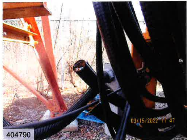
Transmission Lines - Description
