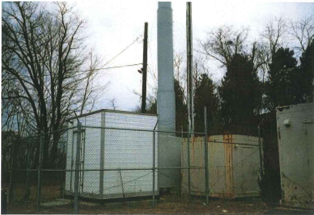
View of the equipment compound looking to the south.
