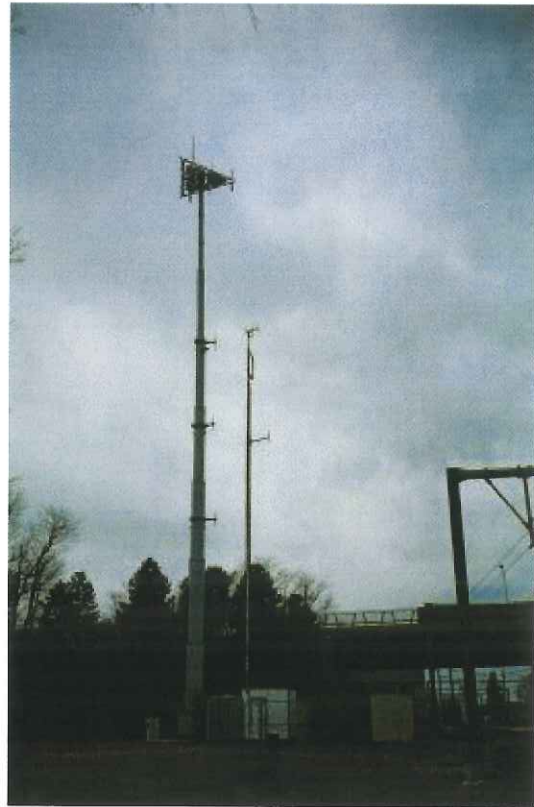
Views of the tower and equipment compound looking west along the railroad tracks.
