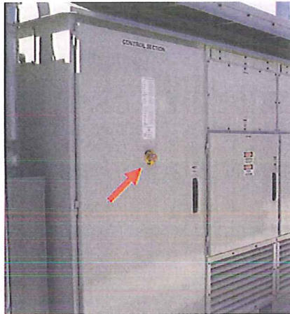
Electrical Balance of Plant
