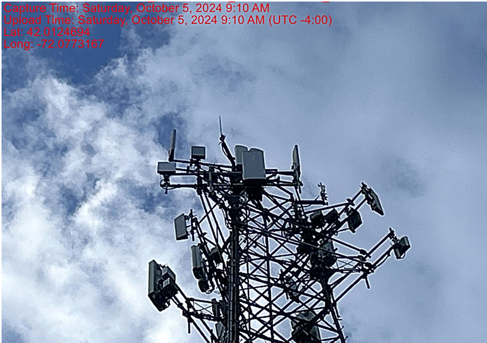
Alpha sector antennas and RRH installed on new sector frame
