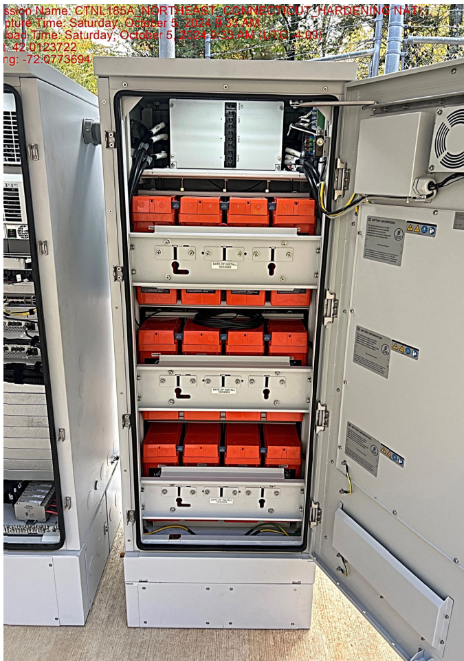
New battery cabinet
