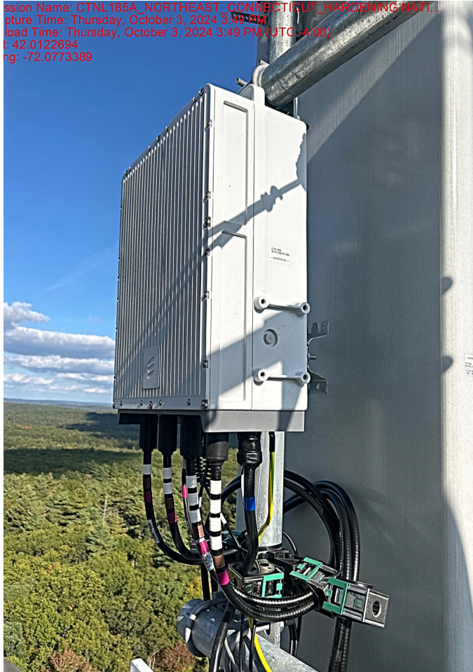
Typical antenna and RRH installation
