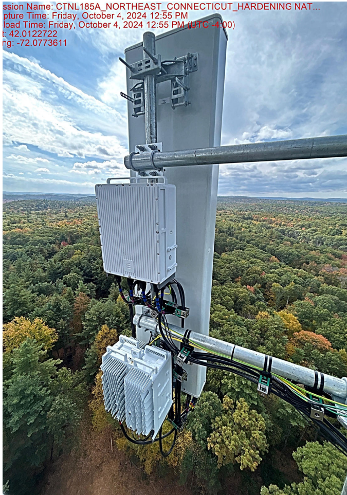
Typical antenna and RRH installation
