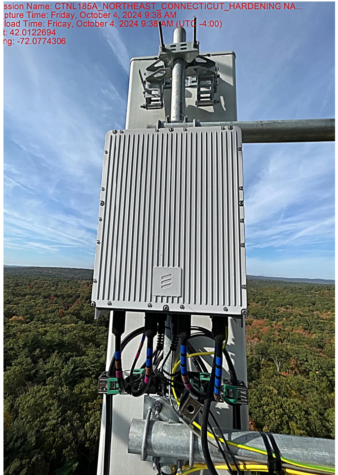
Typical antenna and RRH installation
