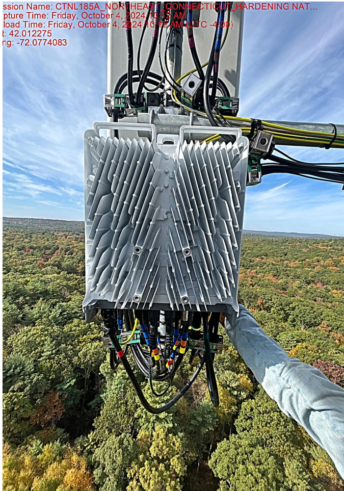
Typical antenna and RRH installation
