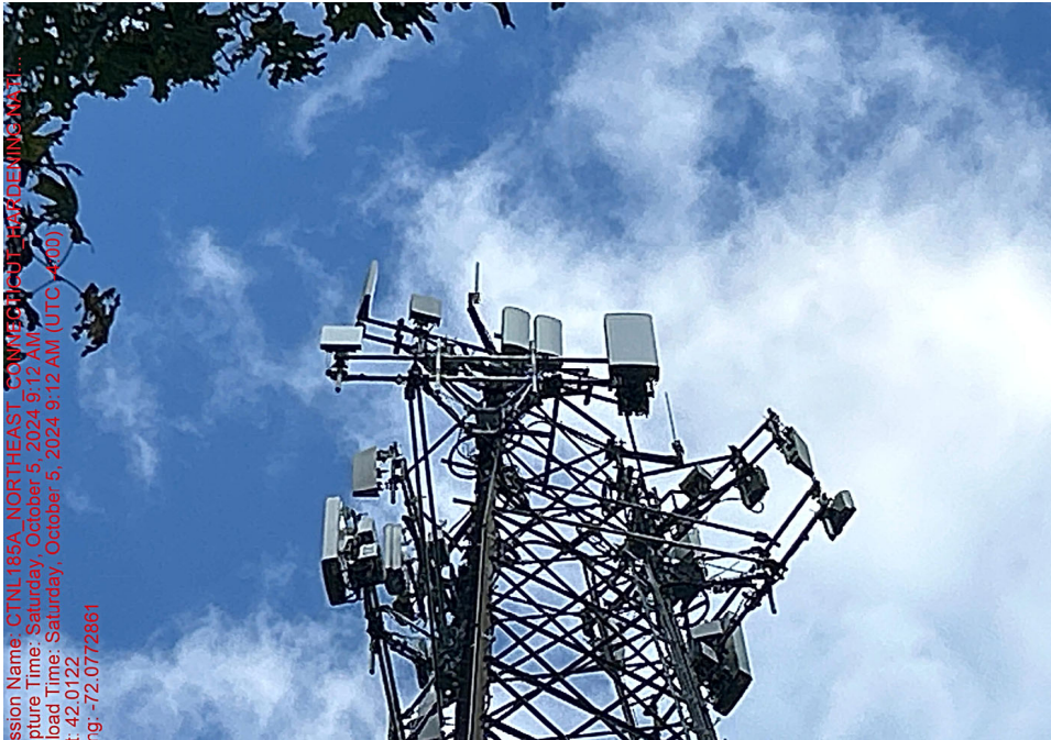
Beta sector antennas and RRH installed on new sector frame
