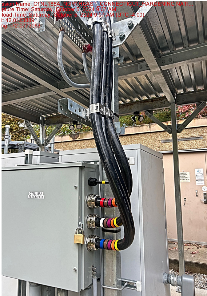
New slack box for cable management
