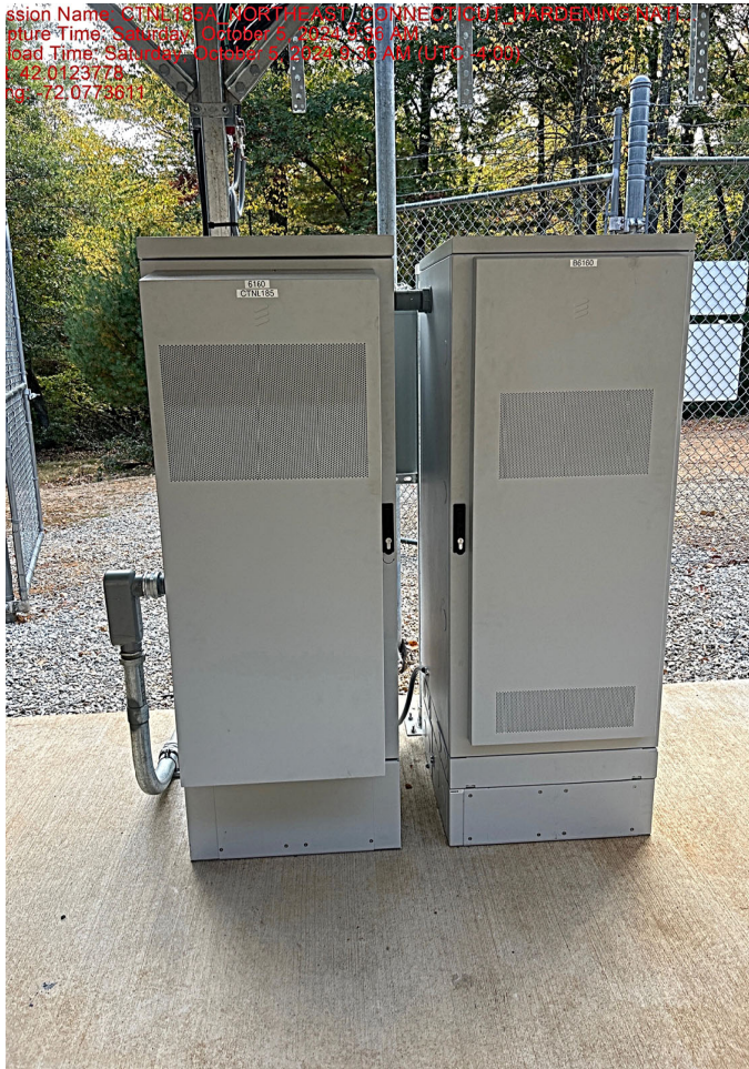
New equipment cabinets mounted to concrete pad
