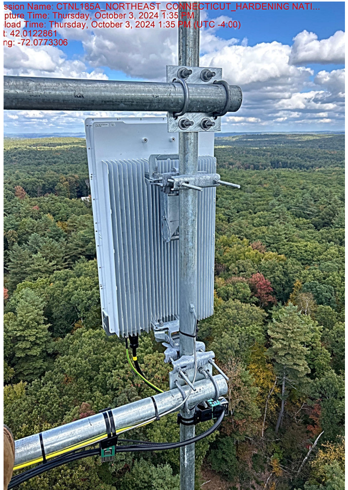
Typical antenna and RRH installation
