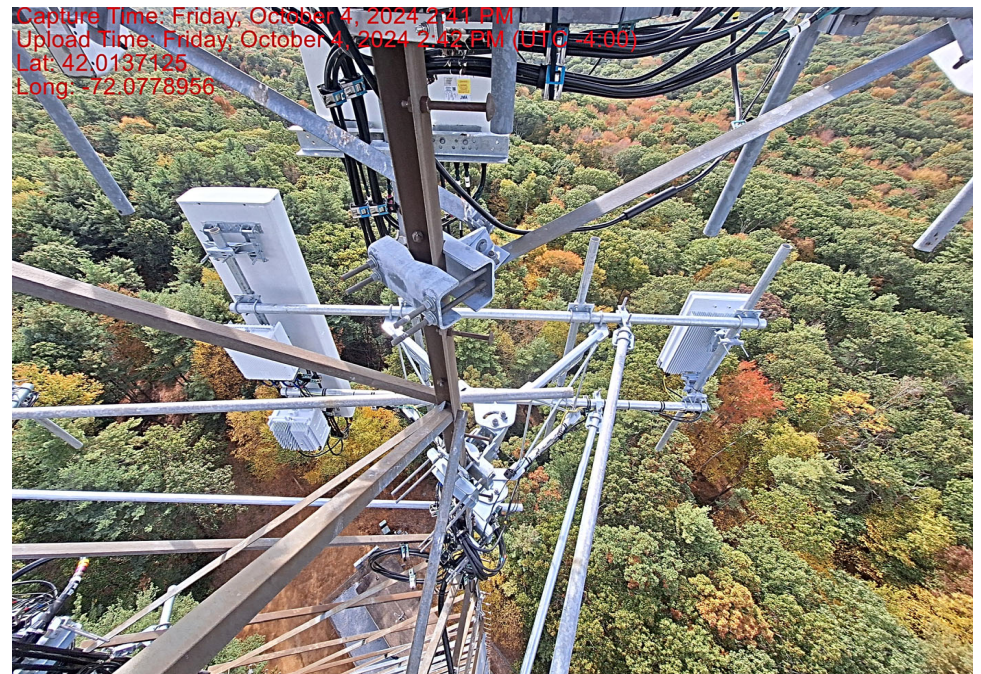
Gamma sector antennas and RRH installed on new sector frame
