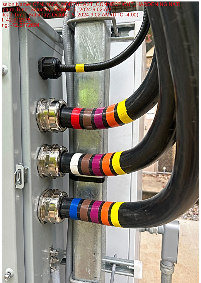
Cable entry at new slack box
