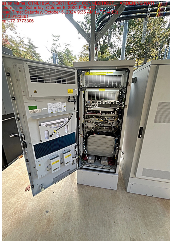
New site support cabinet
