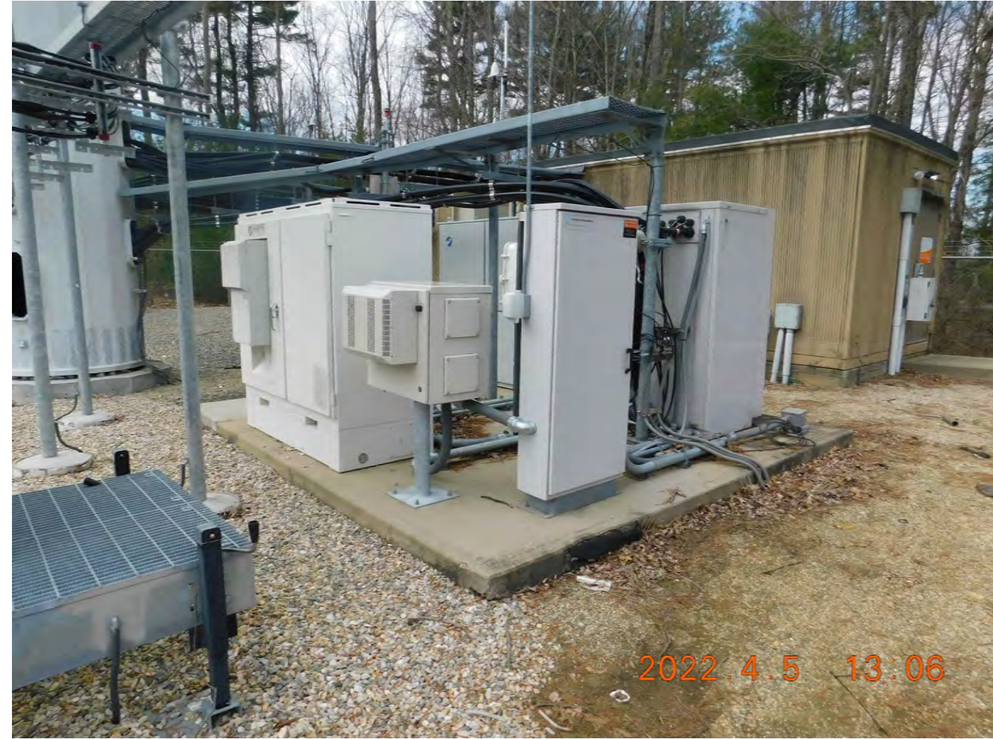
EXISTING EQUIPMENT PHOTO DETAIL SCALE: NTS
