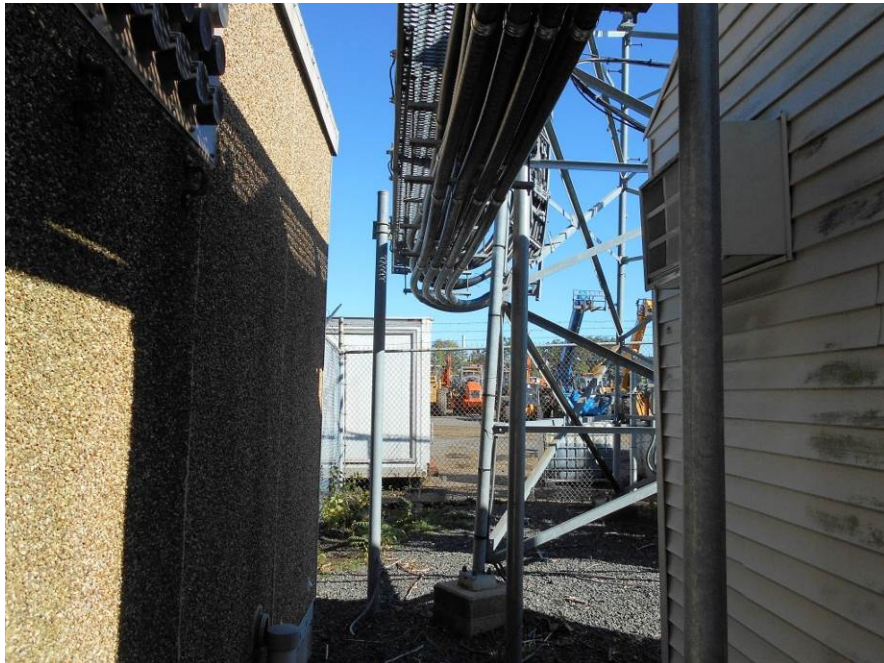
Photo of Verizon's existing ice bridge.
