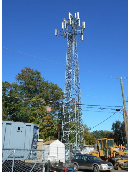
Overview photo of the existing 100' self-supporting tower structure located in Windsor Locks, Connecticut.
