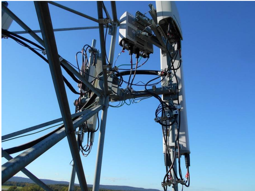
Photo of AT&T's typical existing equipment and mounts at 97'.
