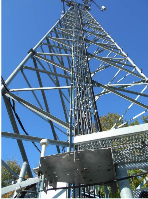
Photo of AT&T's existing waveguide ladder on tower.
