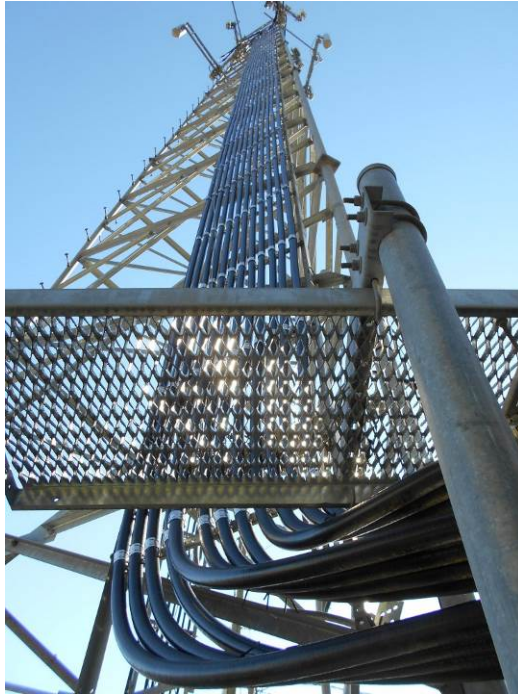
Photo of Verizon's existing waveguide ladder on tower.
