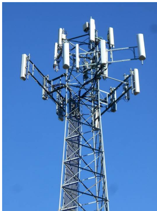
Photo of typical existing equipment and mounts.
