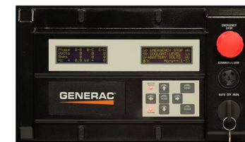
Digital H Control Panel- Dual 4x20 Display
