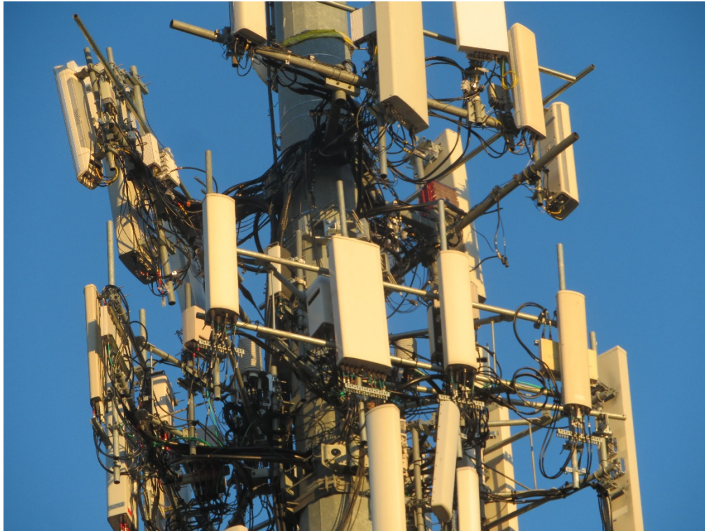
Photo 1: Photo illustrating the Tower with Appurtenances shown.
