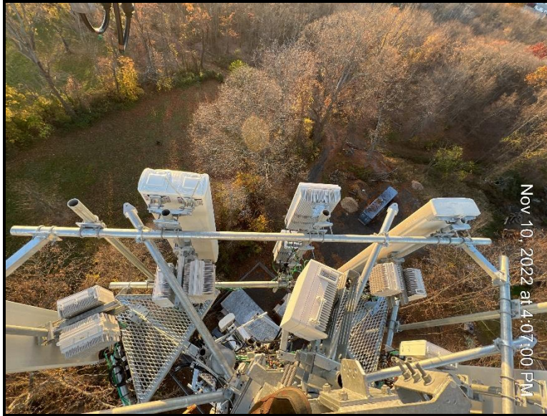
Figure 3: View(s) of installed gamma sector antennas and RRUs on new mount.
