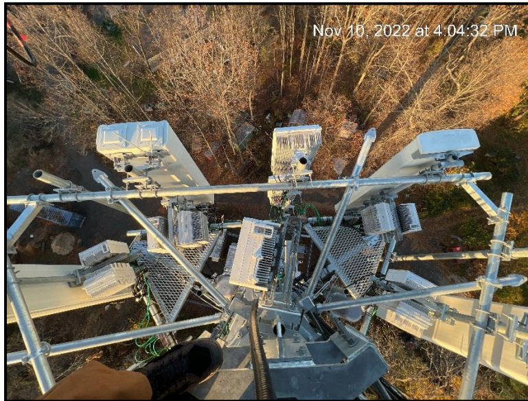
Figure 1: View(s) of installed alpha sector antennas and RRUs on new mount.
