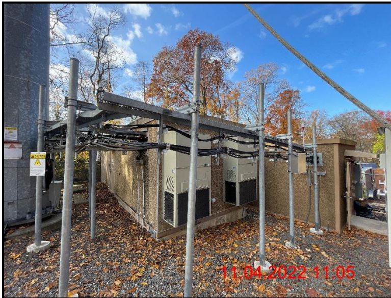
Figure 4: View(s) of installed DC and Fiber trunk cables.
