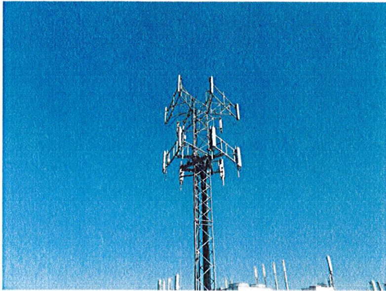
Photo 1: Sample photo of guyed tower on the roof.
