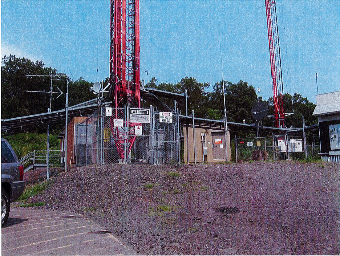
Figure 3: Talcott 2 Compound Facility
