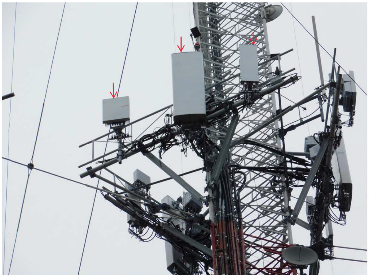
Alpha Sector: (3) New Antennas, (3) New RRHs & Ancillary Equipment Mounted To Modified Sector Frame
