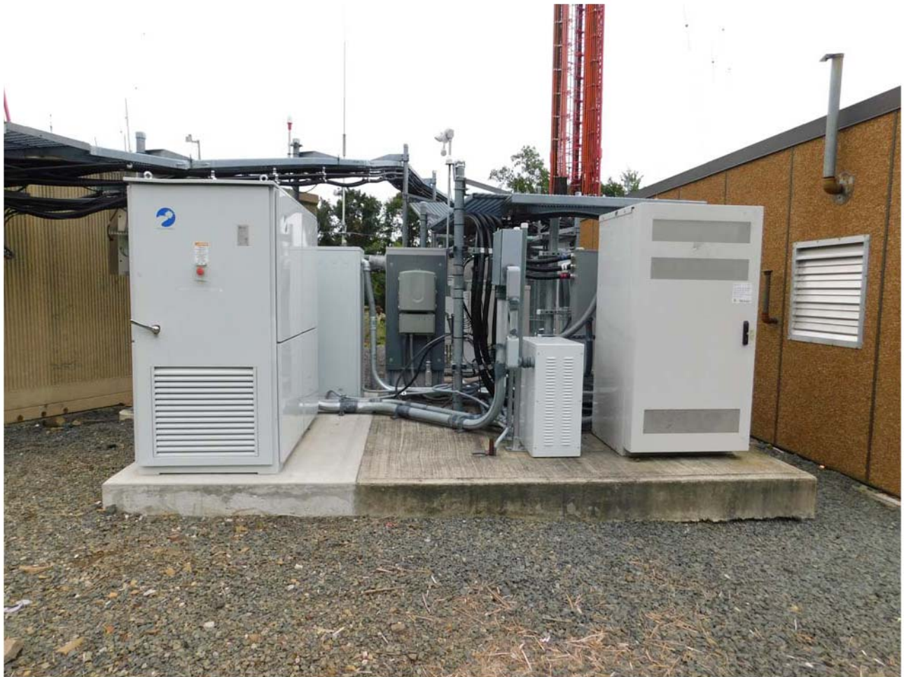
T-Mobile Equipment Mounted To Concrete Pad
