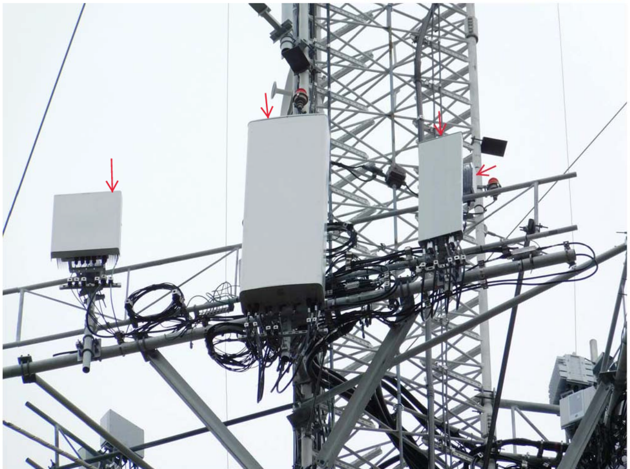
Gamma Sector: (2) New Antennas, (3) New RRHs & Ancillary Equipment Mounted To Modified Sector Frame
