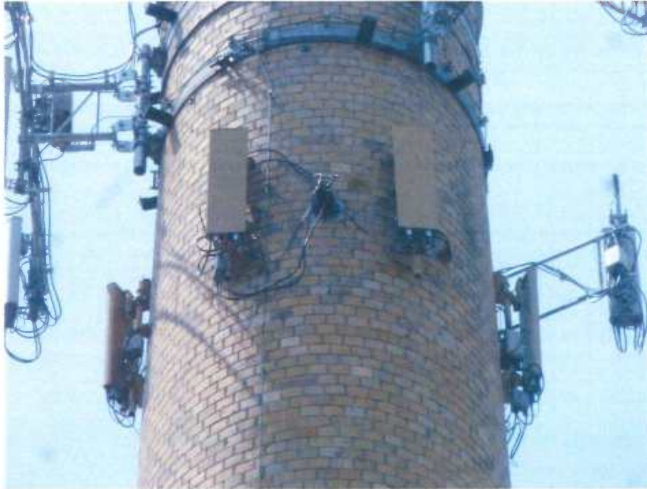
Photo 1: Sample photo illustrating the existing T-Mobile antennas.
