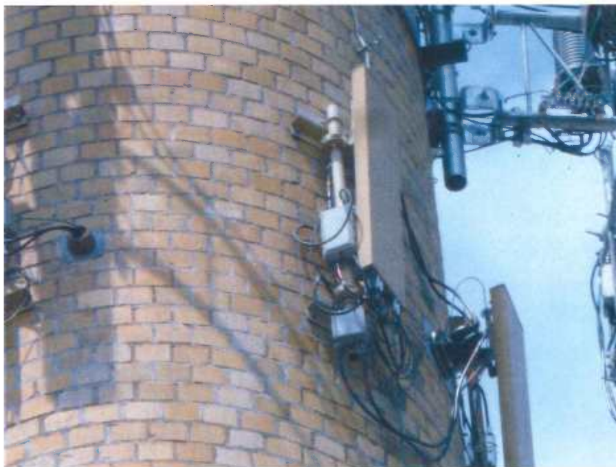
Photo 2: Sample photo illustrating the connection of the T-Mobile antennas to the face of the smokestack.
