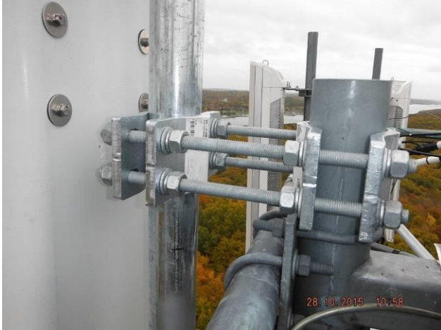
New pipe mount attachment to existing sector frame (photo provided by contractor)
