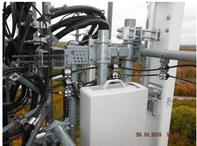
RRU pipe mount attachment to sector frame (photo provided by contractor)
