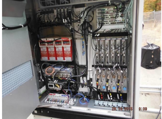
RAN equipment within 3106 cabinet (photo provided by contractor)
