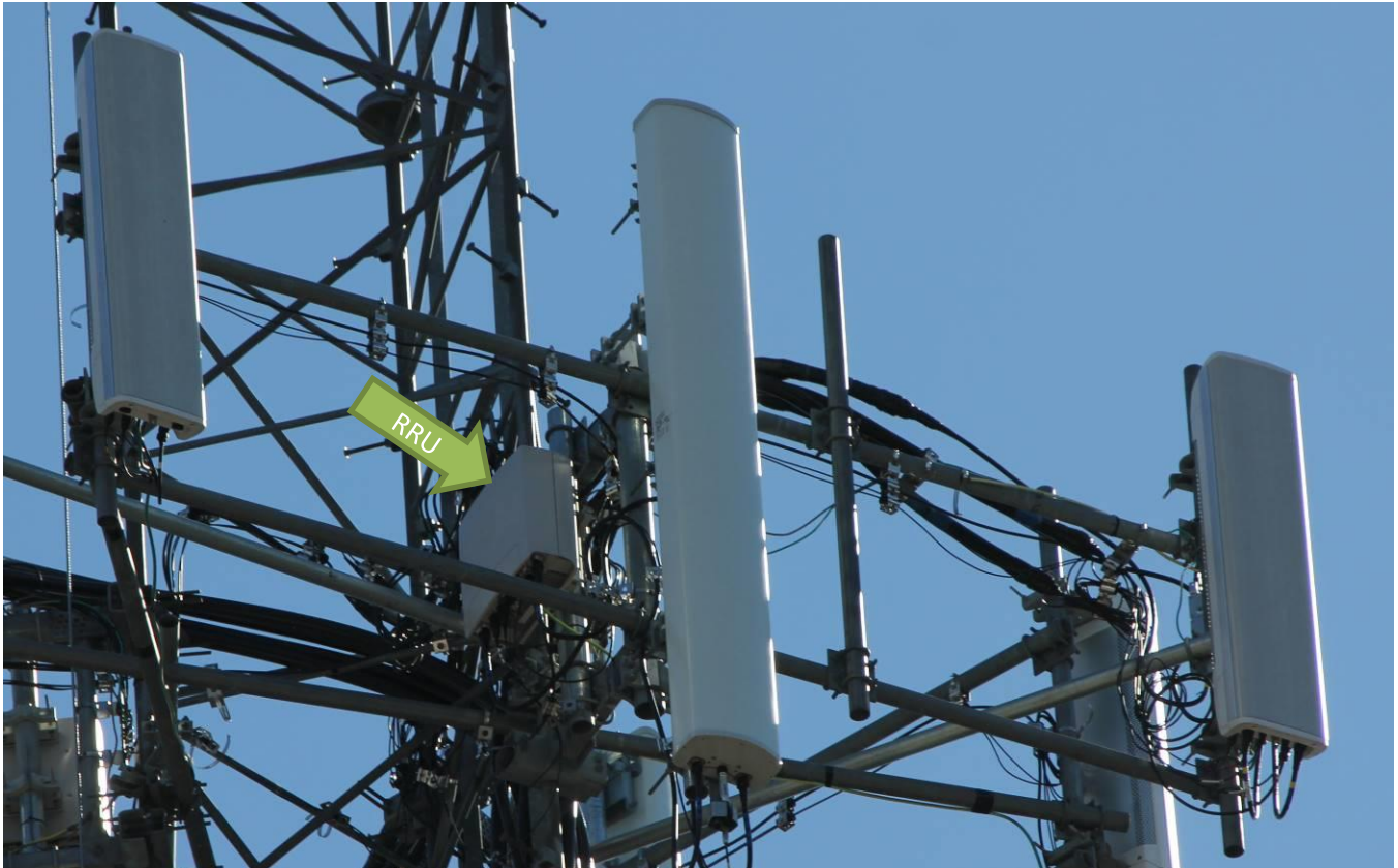
Typical sector showing new panel antenna and RRU (center) and existing panel antennas (left and right)
