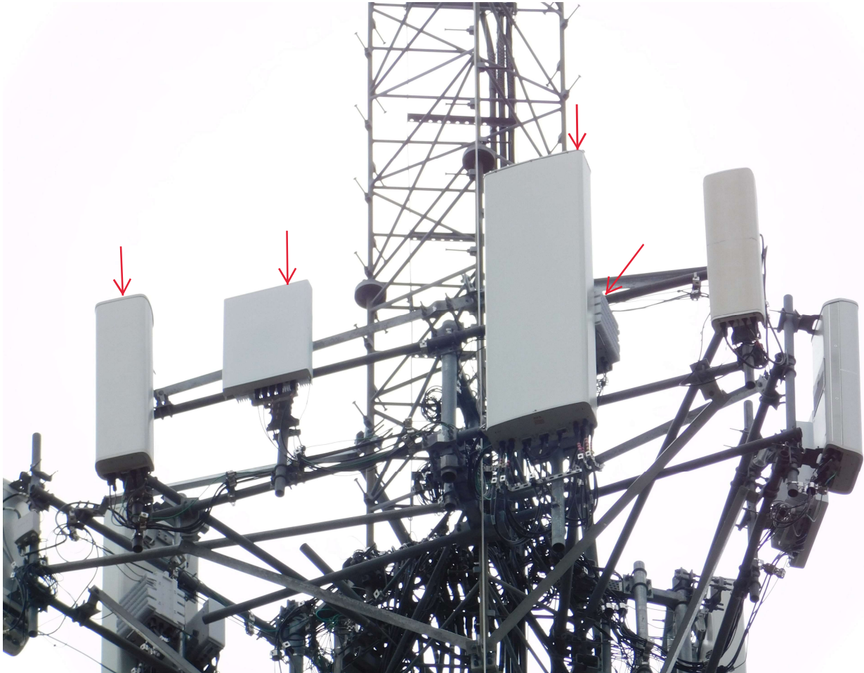
Alpha Sector: (3) New Antennas & (2) New RRHs Mounted To Modified Sector Frame
