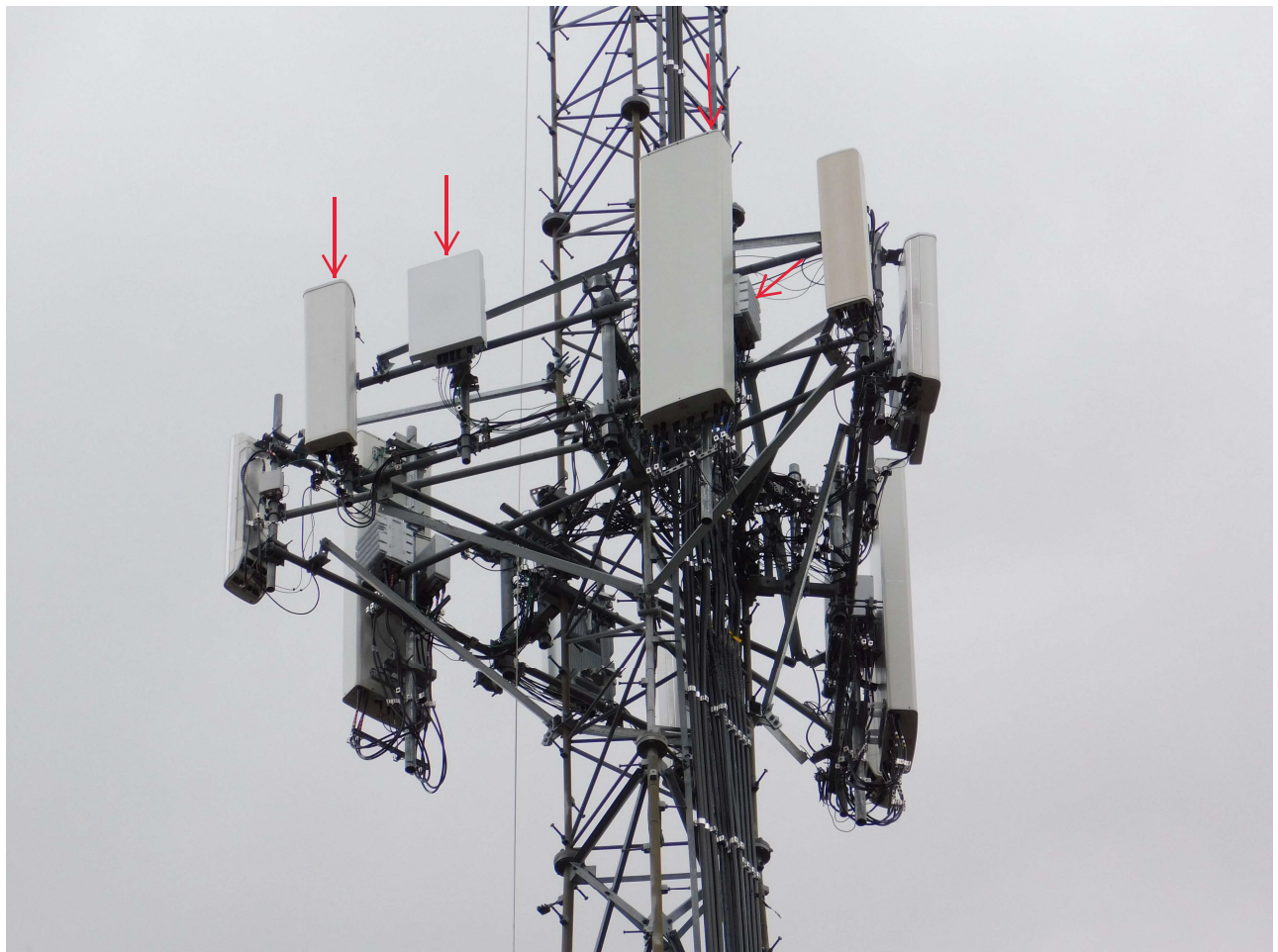
Gamma Sector: (3) New Antennas & (2) New RRHs Mounted To Modified Sector Frame
