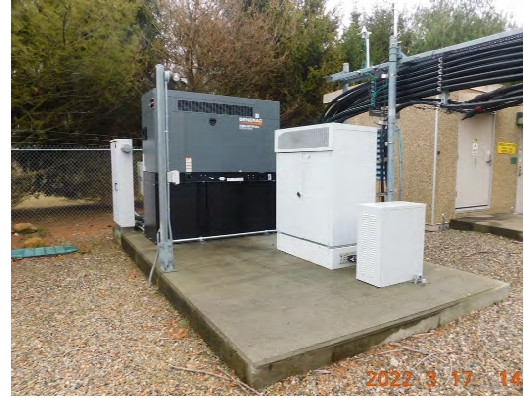
EXISTING EQUIPMENT PHOTO DETAIL SCALE: NTS
