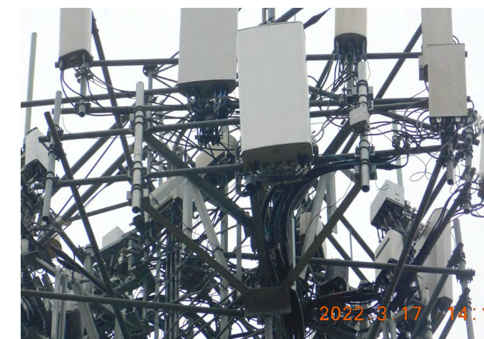
EXISTING ANTENNA ARRAY
