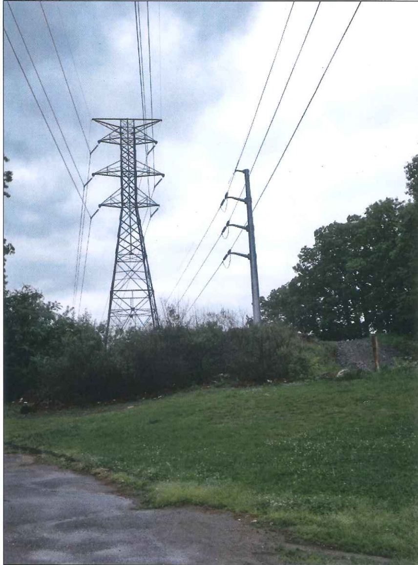
View of the transmission towers from west, from access location
