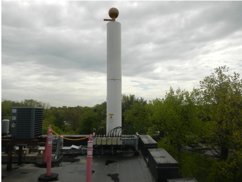
EXISTING RF TRANSPARENT CANISTER AND SUPPORTING STEEL PLATFORM ON ROOF
