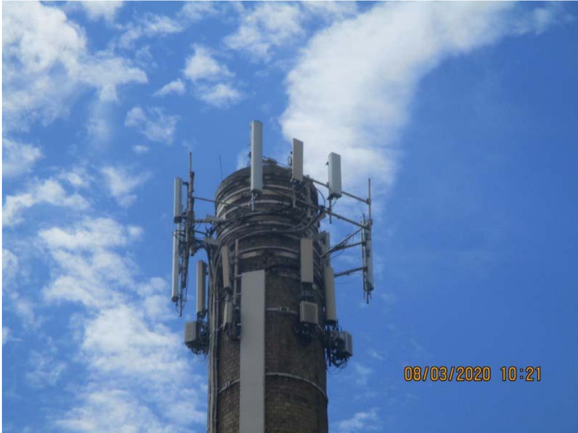
Existing smokestack and sector mounts
