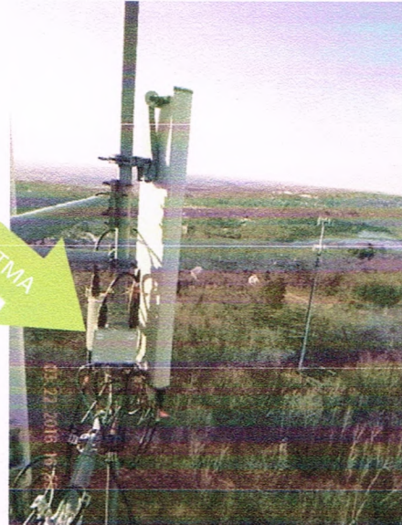
AFTER - TMAs Behind Antenna Contractor Photo
