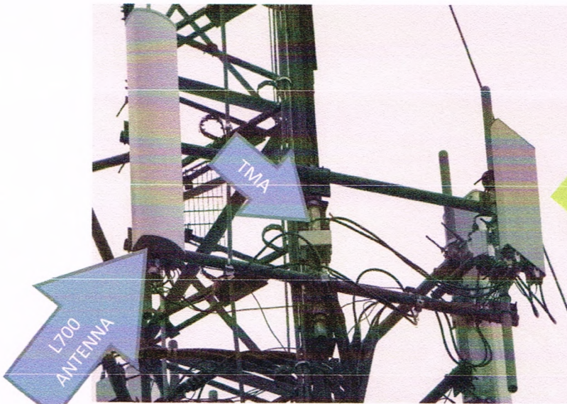
BEFORE - Photo, TMAs in center position
