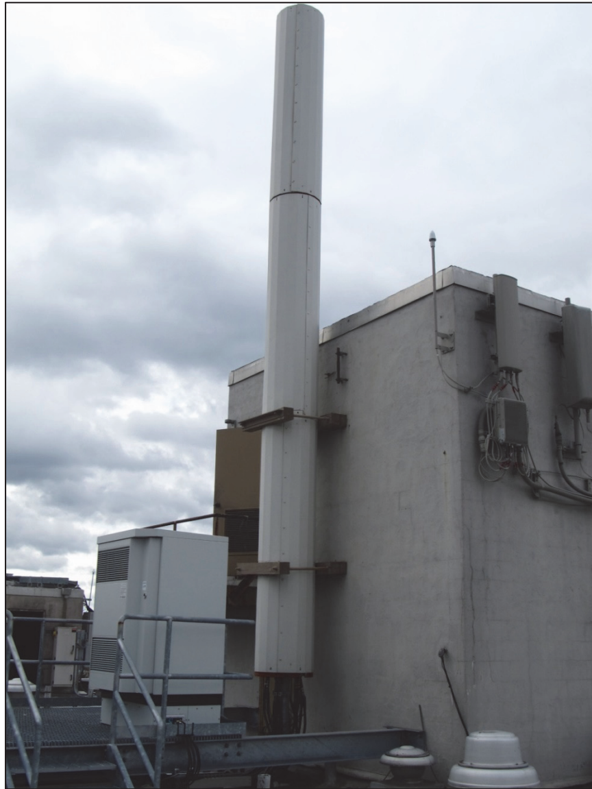
Existing Antennas inside the Stealth Canister Pole
