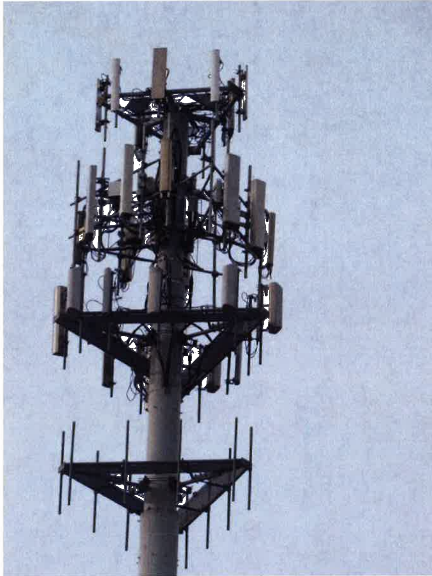
Photo 1: Photo illustrating the Monopole with Appurtenances shown.
