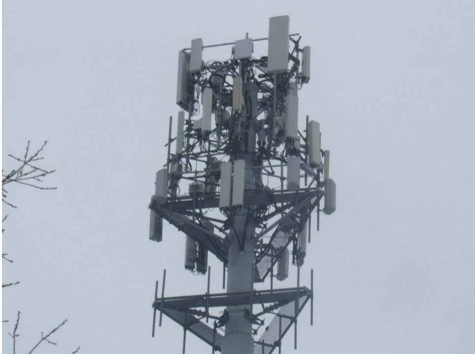
Photo 1: Photo illustrating the Tower with Appurtenances shown.
