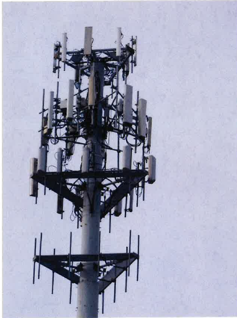
Photo 1: Photo illustrating the Monopole with Appurtenances shown.
