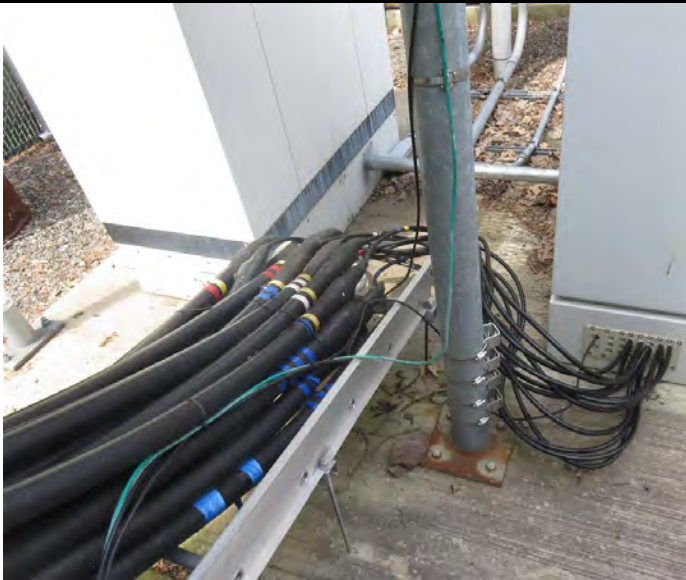
COAX ROUTING TO T-MOBILE
