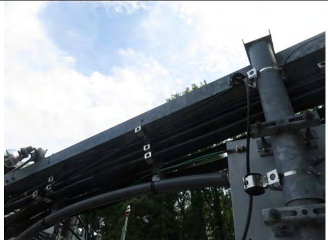
COAX ROUTING AT&T
