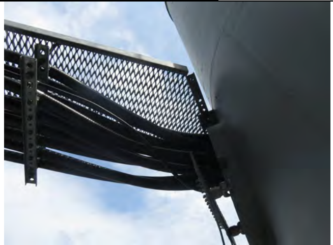
COAX ROUTING TO SHELTER A
