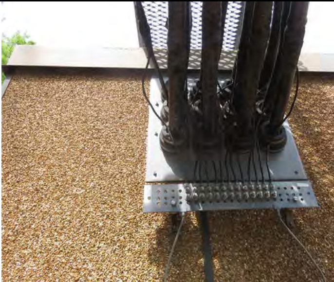
COAX ROUTING TO SHELTER A
