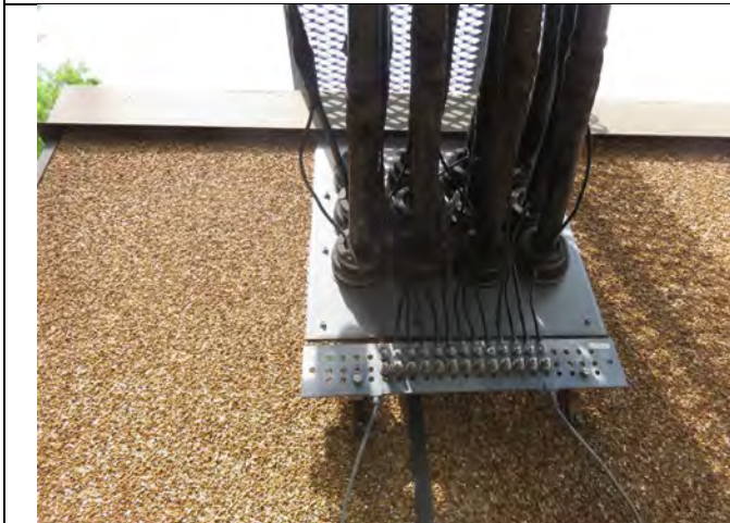
COAX ROUTING TO SHELTER A
