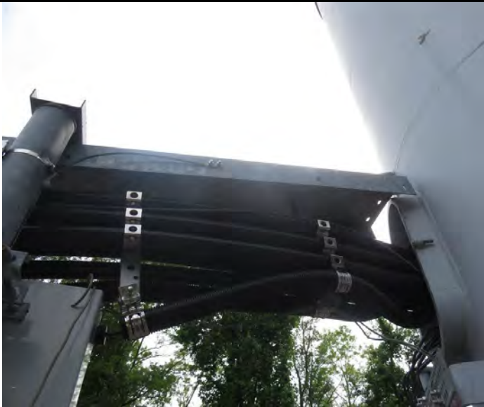
COAX ROUTING AT&T
