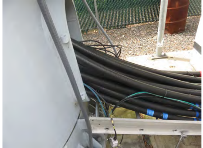
COAX ROUTING TO T-MOBILE
