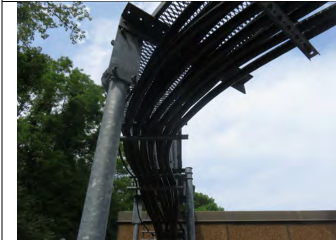
COAX ROUTING TO SHELTER A
