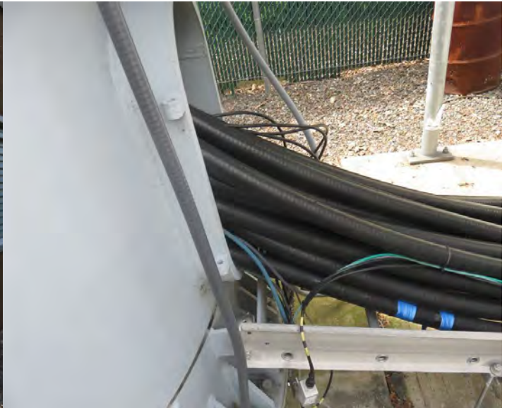
COAX ROUTING TO T-MOBILE
