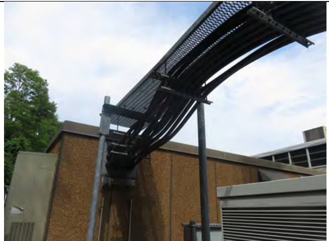
COAX ROUTING TO SHELTER A
