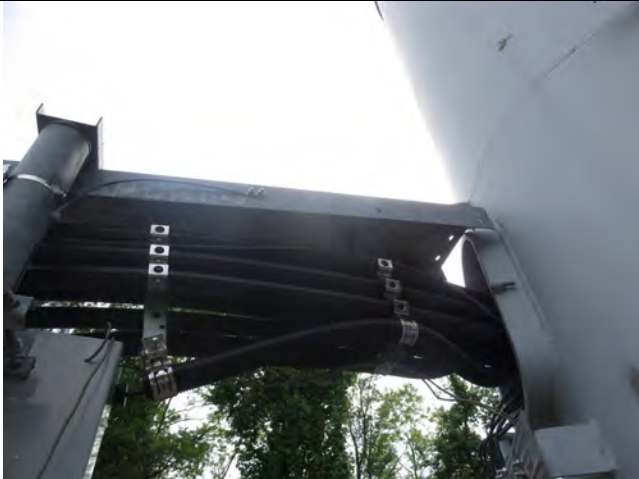
COAX ROUTING AT&T
