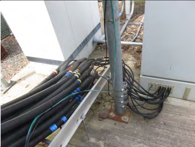
COAX ROUTING TO T-MOBILE
