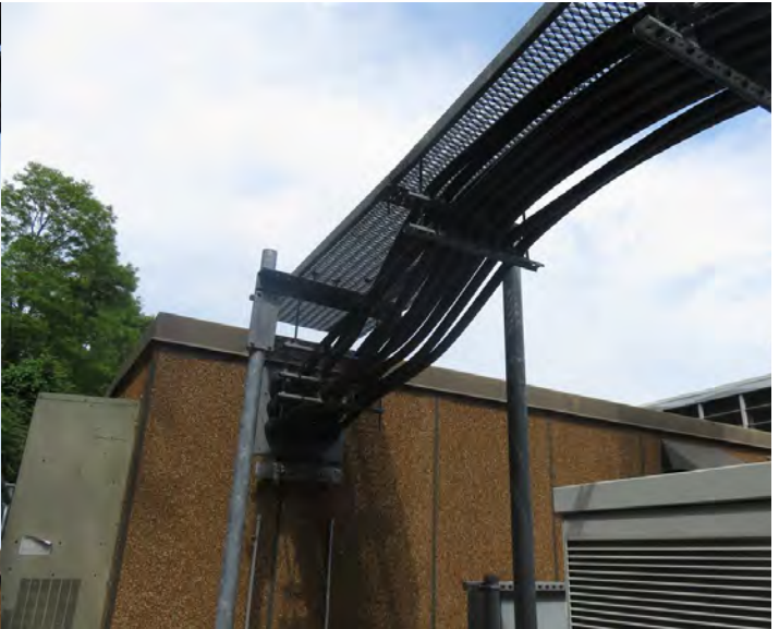
COAX ROUTING TO SHELTER A
