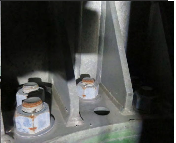
INSIDE TOWER JOINT 2 MISSING BOLT
