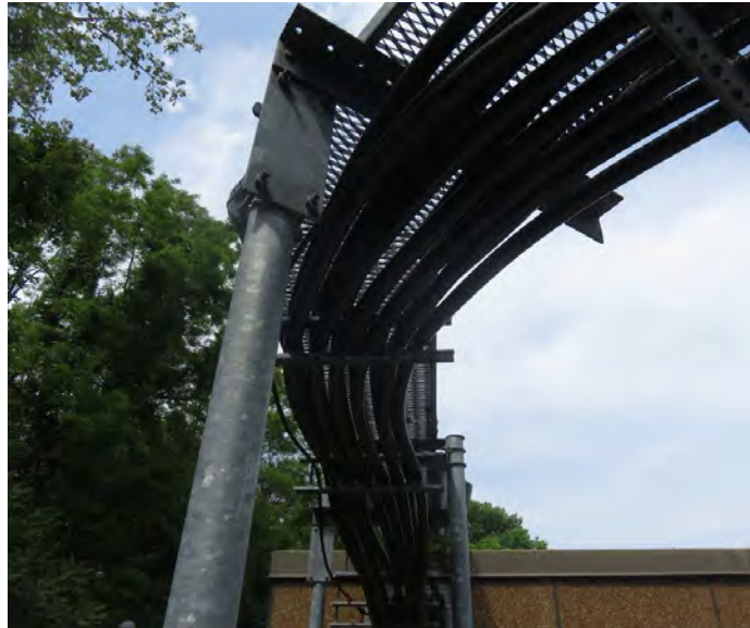
COAX ROUTING TO SHELTER A
