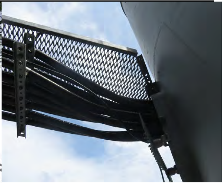
COAX ROUTING TO SHELTER A
