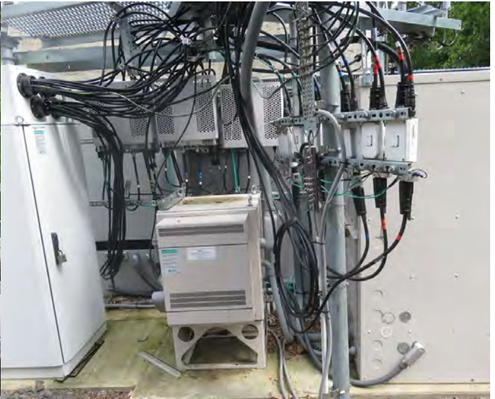
COAX ROUTING AT&T
