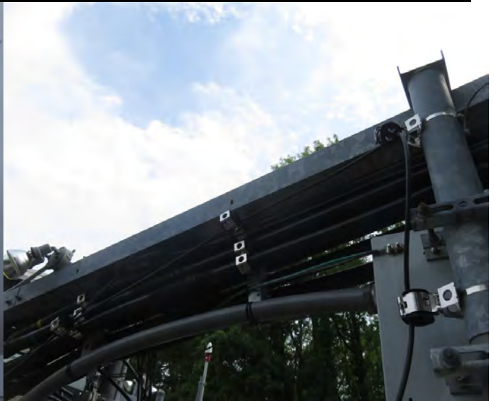
COAX ROUTING AT&T
