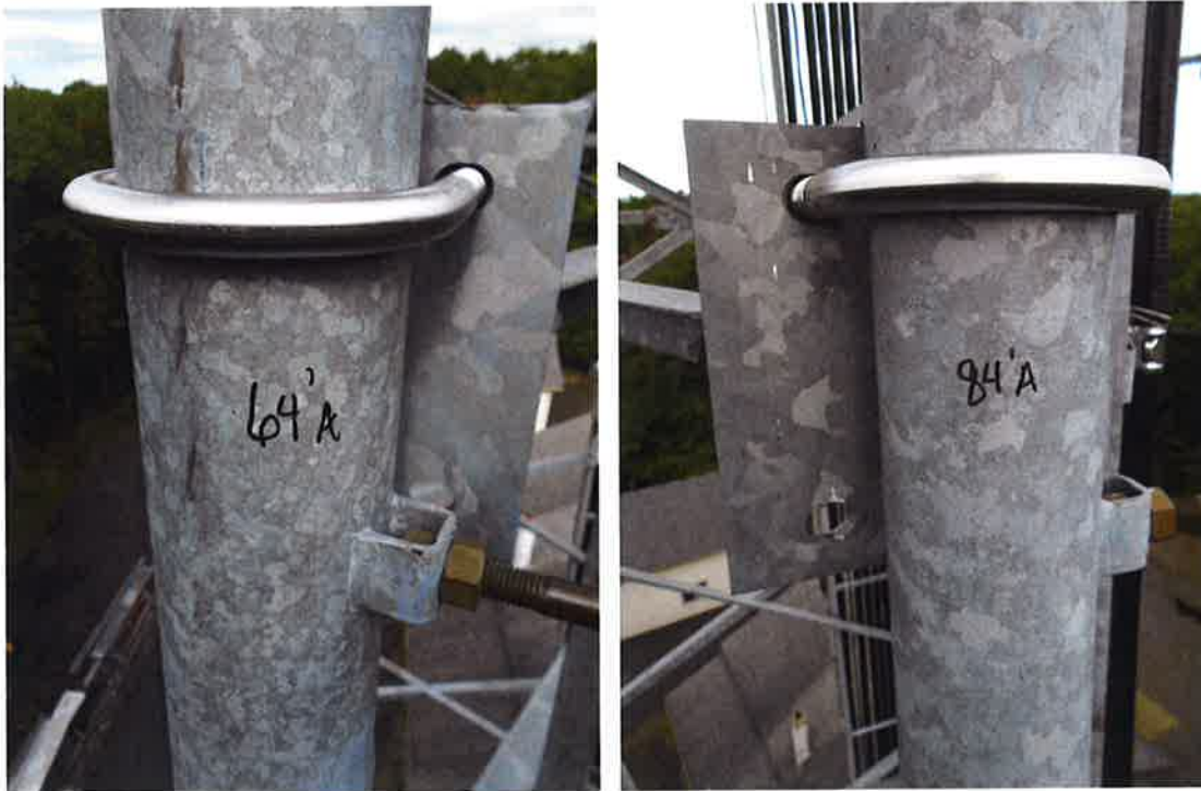
Photos of missing U-bolts at 64' and 84'.
