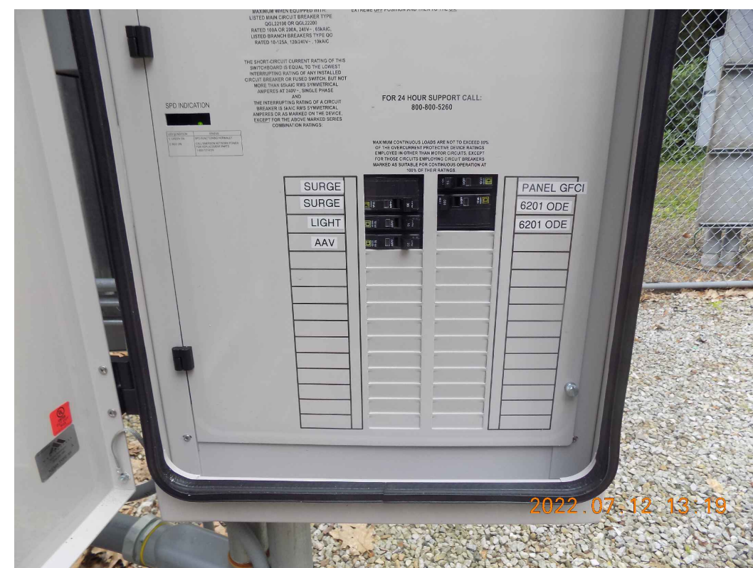
EXISTING POWER PANEL PHOTO SCALE: NOT TO SCALE
