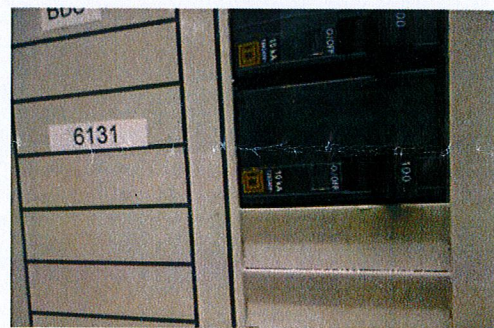
100A-2P breaker for the 3106 equipment cabinet with the 6131 upgrade.
