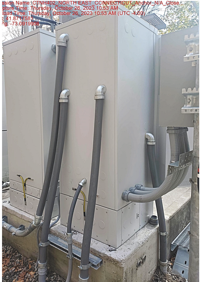
Grounding and conduits installed at rear of cabinets
