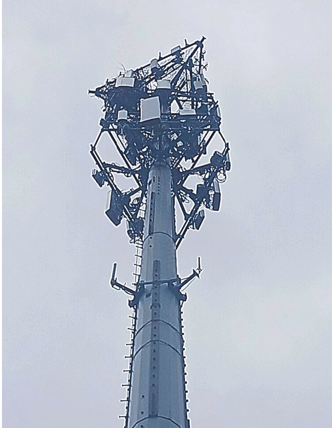
Alpha sector antennas installed on existing mount
