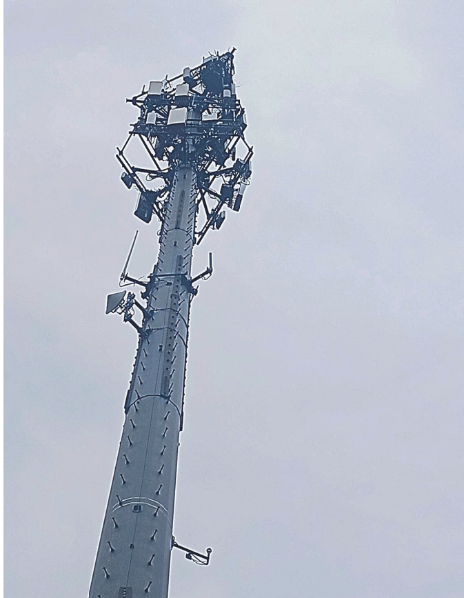
Beta sector antennas installed on existing mount
