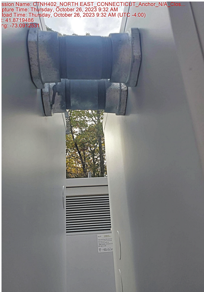
Conduit interconnects between cabinets
