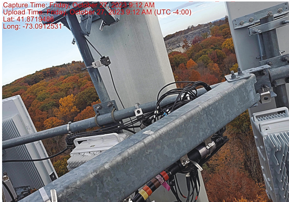
Alpha sector antennas installed on existing mount
