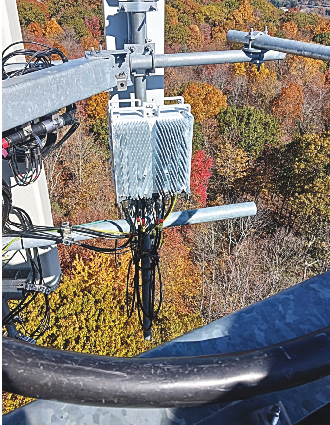
Typical RRH installed on existing mount
