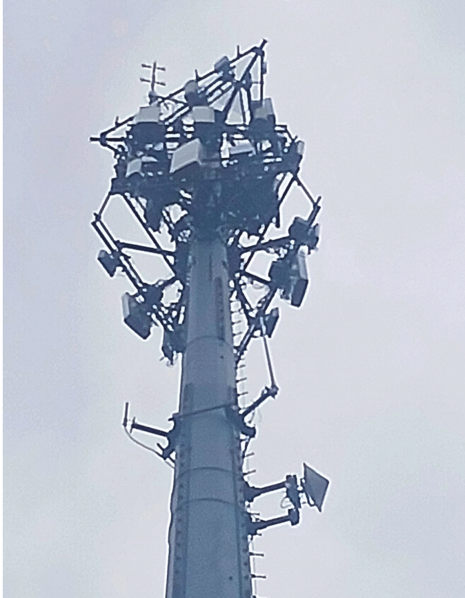
Gamma sector antennas installed on existing mount
