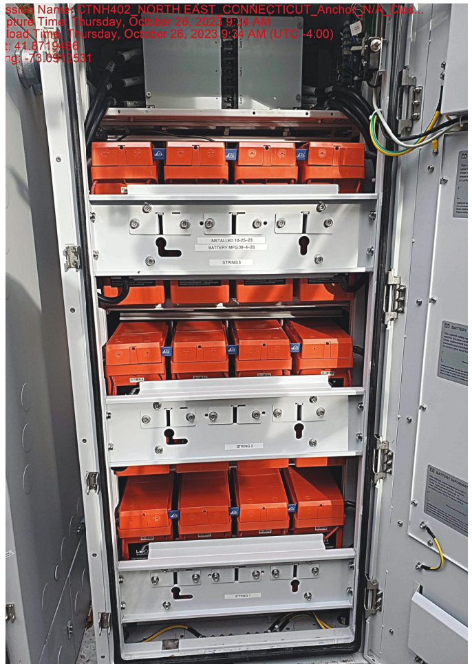
Battery cabinet installed on concrete pad
