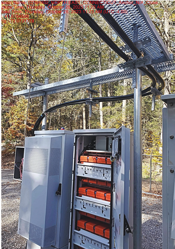
Equipment cabinets installed on concrete pad
