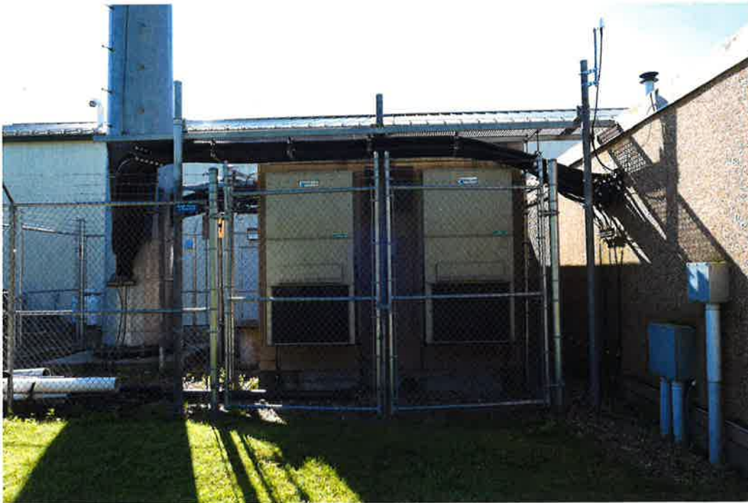
Photo of Verizon's existing feed lines and ice bridge to tower.
