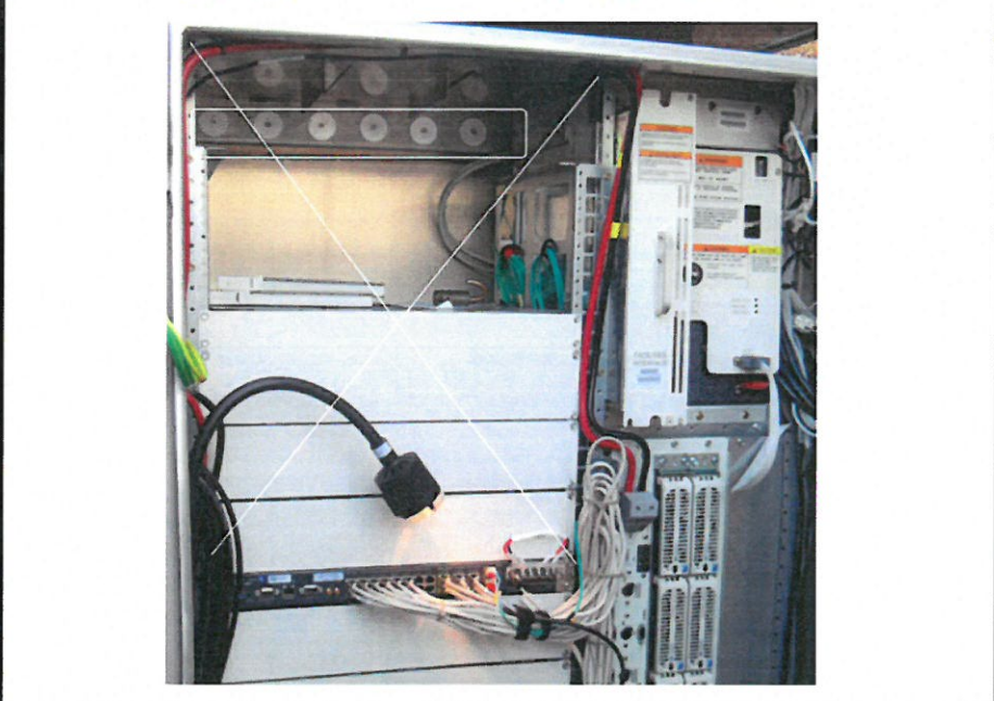
INSIDE MMBTS CABINET
