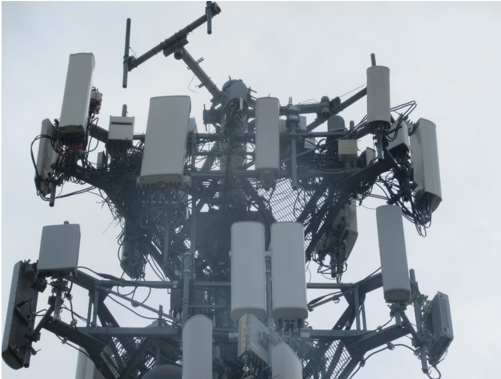
Photo 1: Photo illustrating the Tower with Appurtenances shown.
