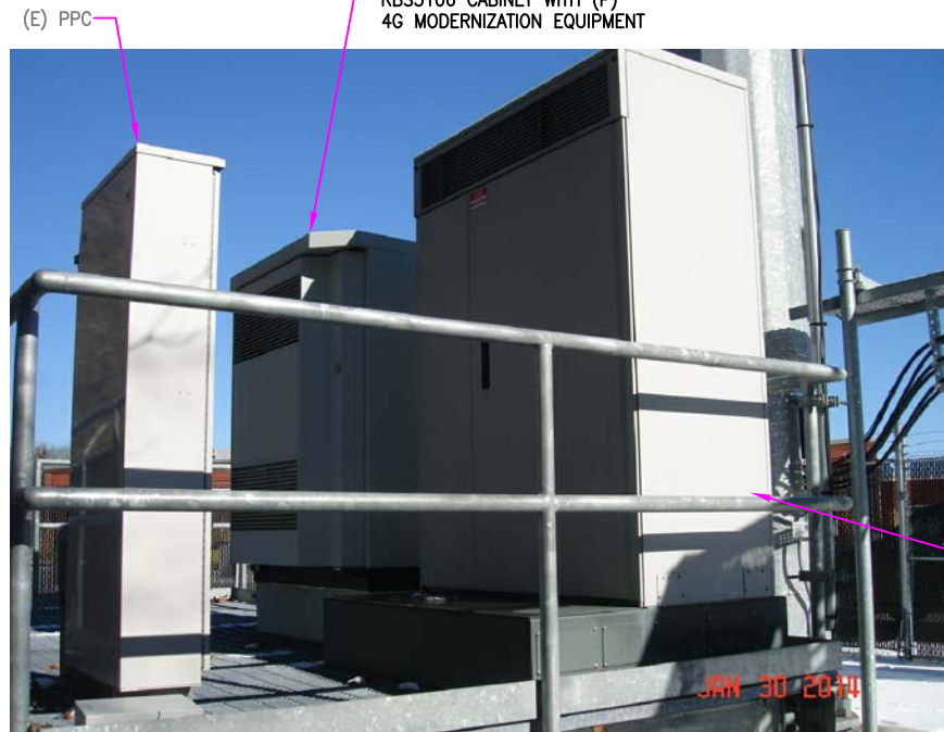
4 EXISTING EQUIPMENT AREA.
