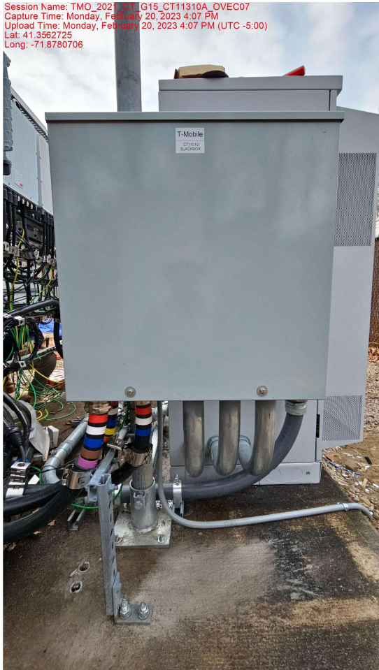
(1) New Slack Box Installed In Existing Equipment Area
