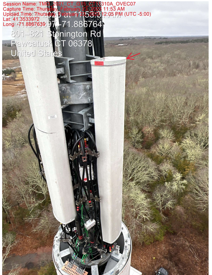
Alpha Sector: (1) New Antenna Mounted To Existing Unipole
