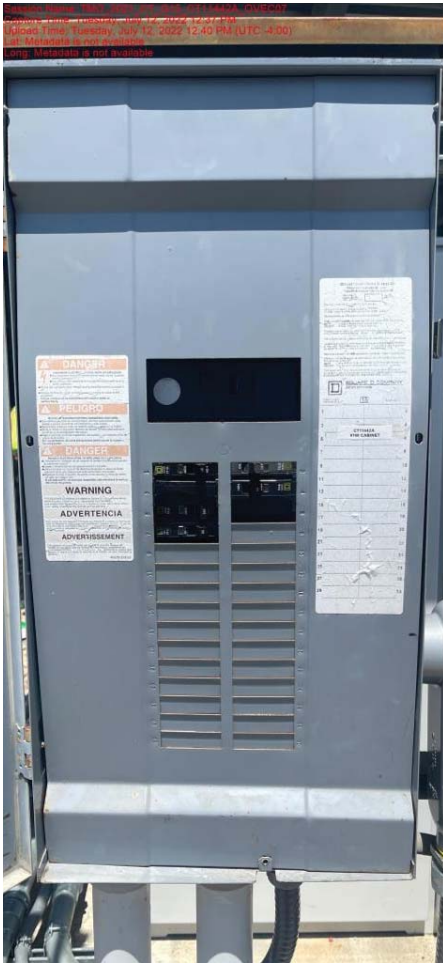
New Equipment Tied Into Existing Electrical Panel
