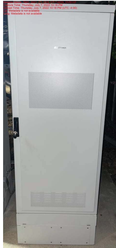
New Battery Cabinet Mounted To Existing Concrete Pad
