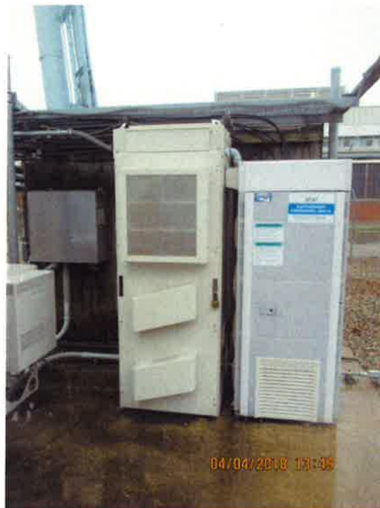
Photo 2: Sample photo illustrating the existing equipment cabinets.
