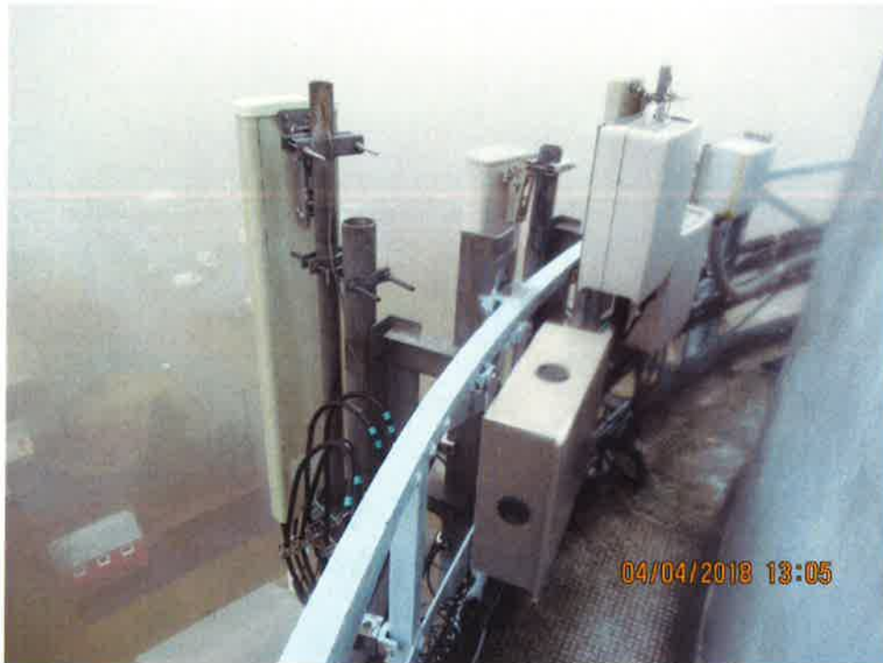
Photo 1: Sample photo illustrating the existing antennas and RRH's.
