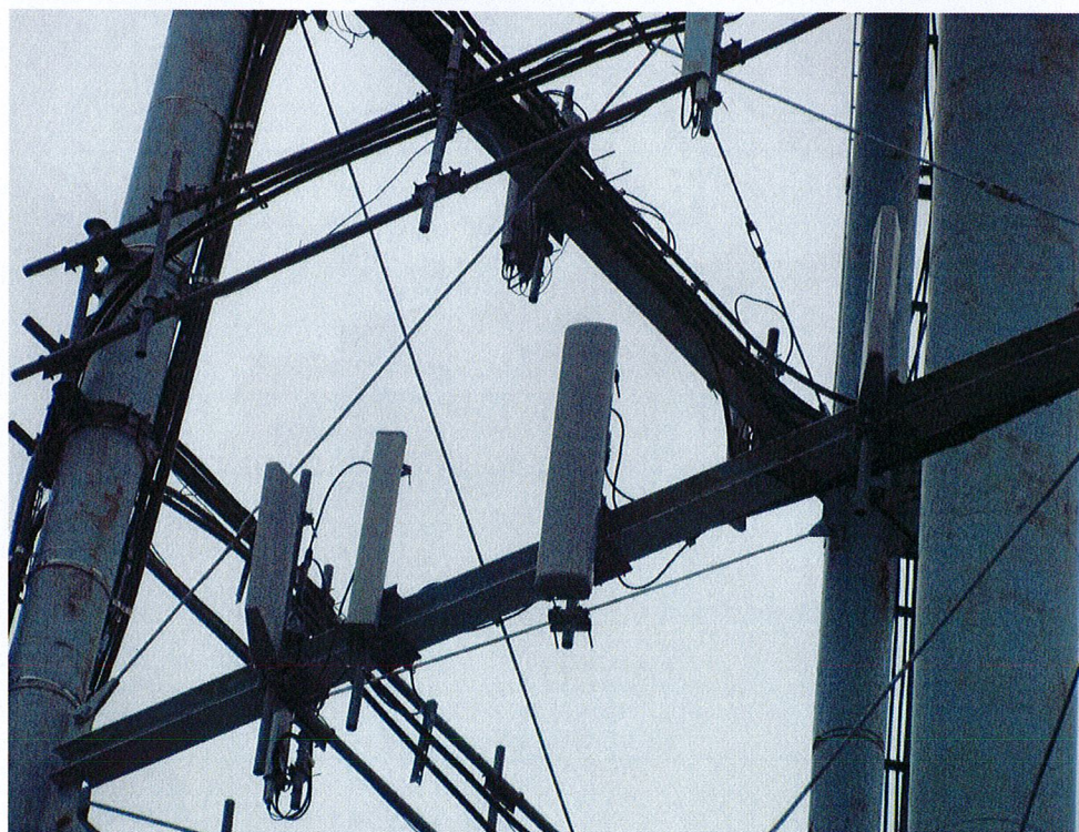
Figure 16: Verizon Wireless Antennas #36 through #39
