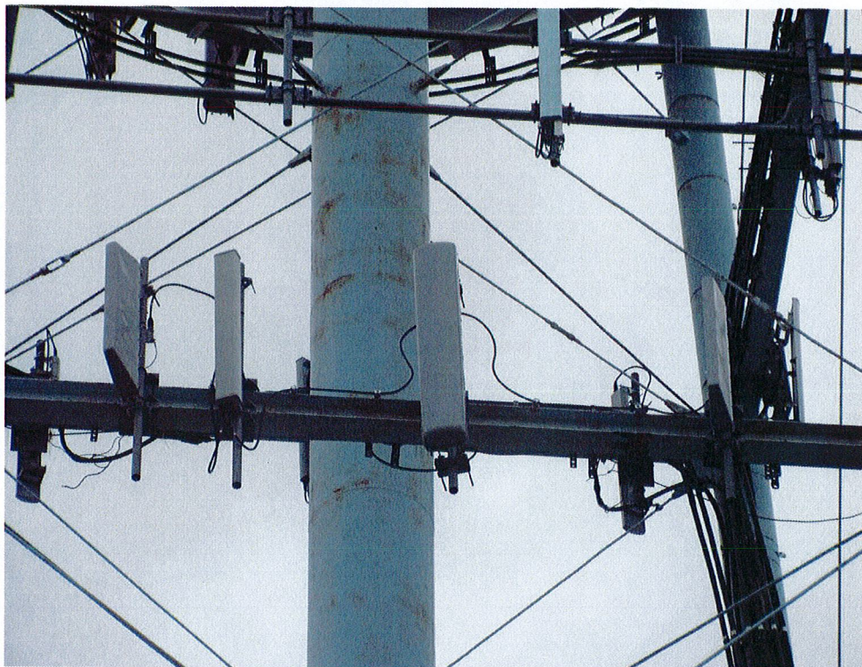
Figure 15: Verizon Wireless Antennas #32 through #35
