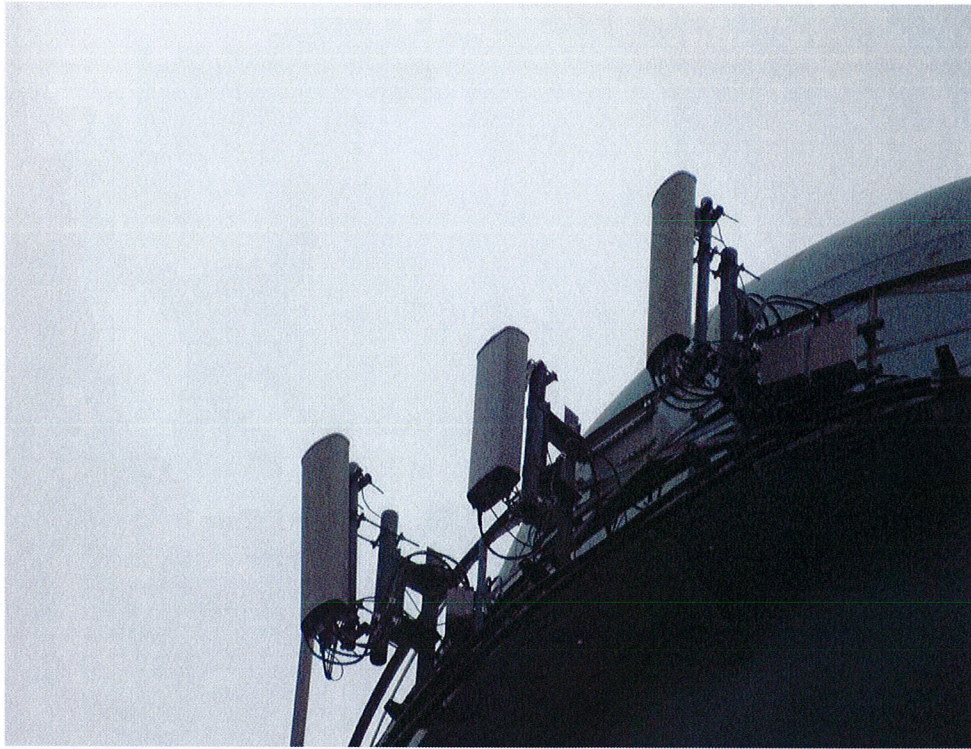
Figure 3: AT&T Mobility, LLC Gamma Sector Antennas #7 through #9
