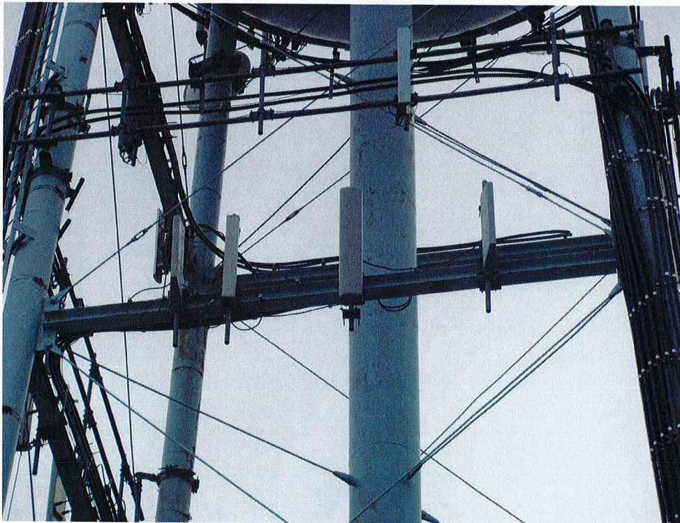
Figure 14: Verizon Wireless Antennas #28 through #31
