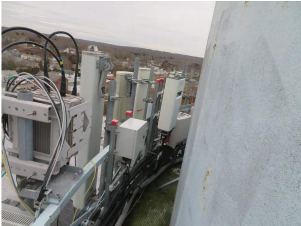
Photo 2: Sample photo illustrating the existing antennas and RRH's.
