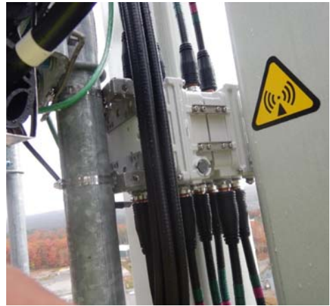
Diplexer installed behind dual-mounted antennas
