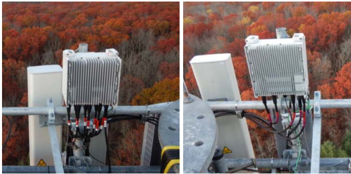
RRH's mounted behind antennas
