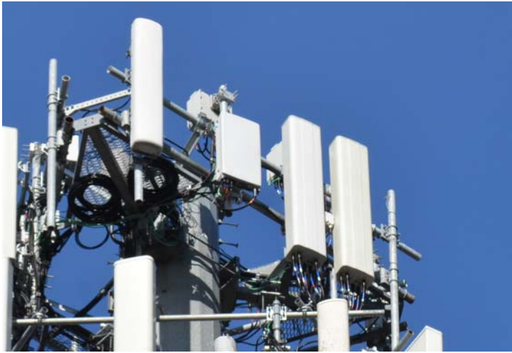
Overall Verizon antenna array
