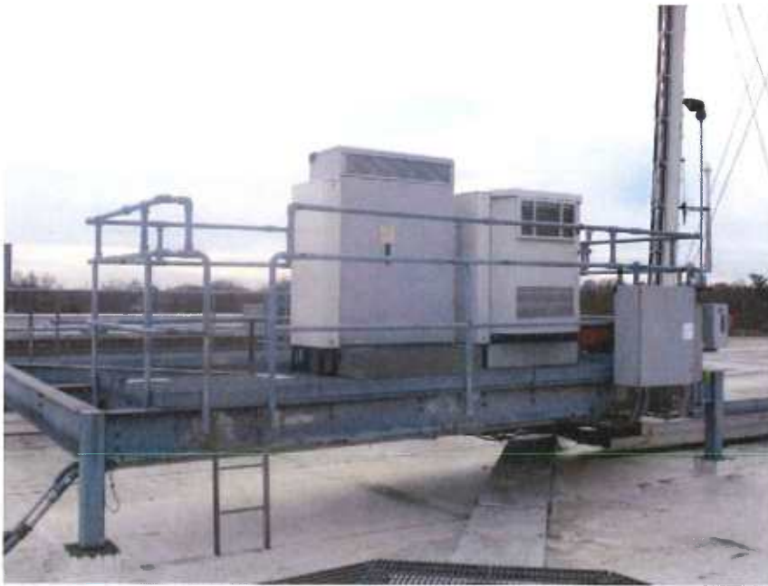
Existing equipment on the Rooftop
