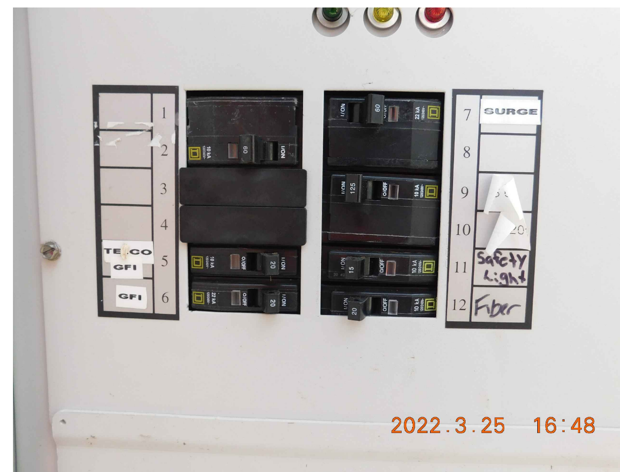
EXISTING POWER PANEL PHOTOS SCALE: NOT TO SCALE
