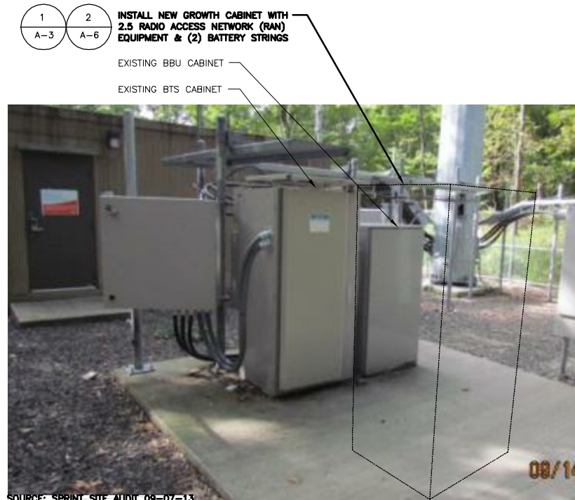
RAN EQUIPMENT PHOTO DETAIL SCALE: N.T.S.
