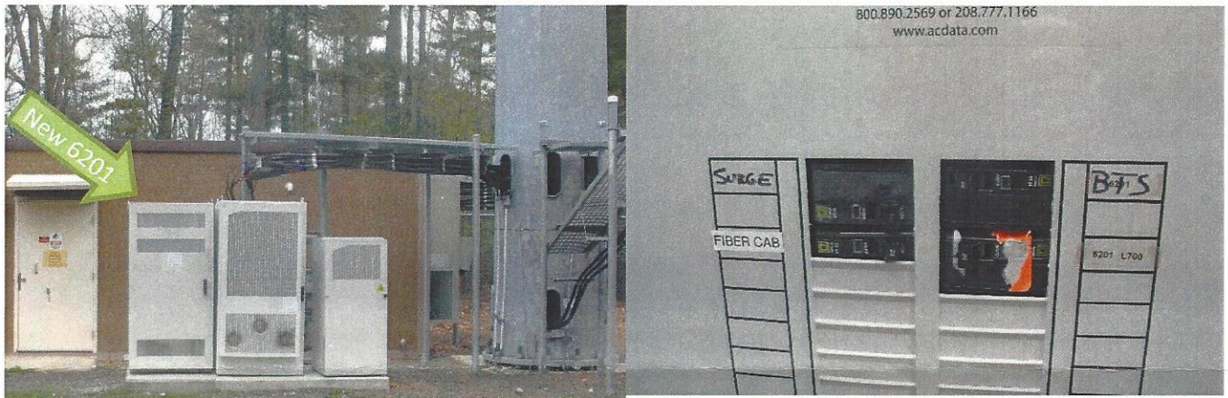
Existing T-Mobile equipment area and new 6201 cabinet (left).
