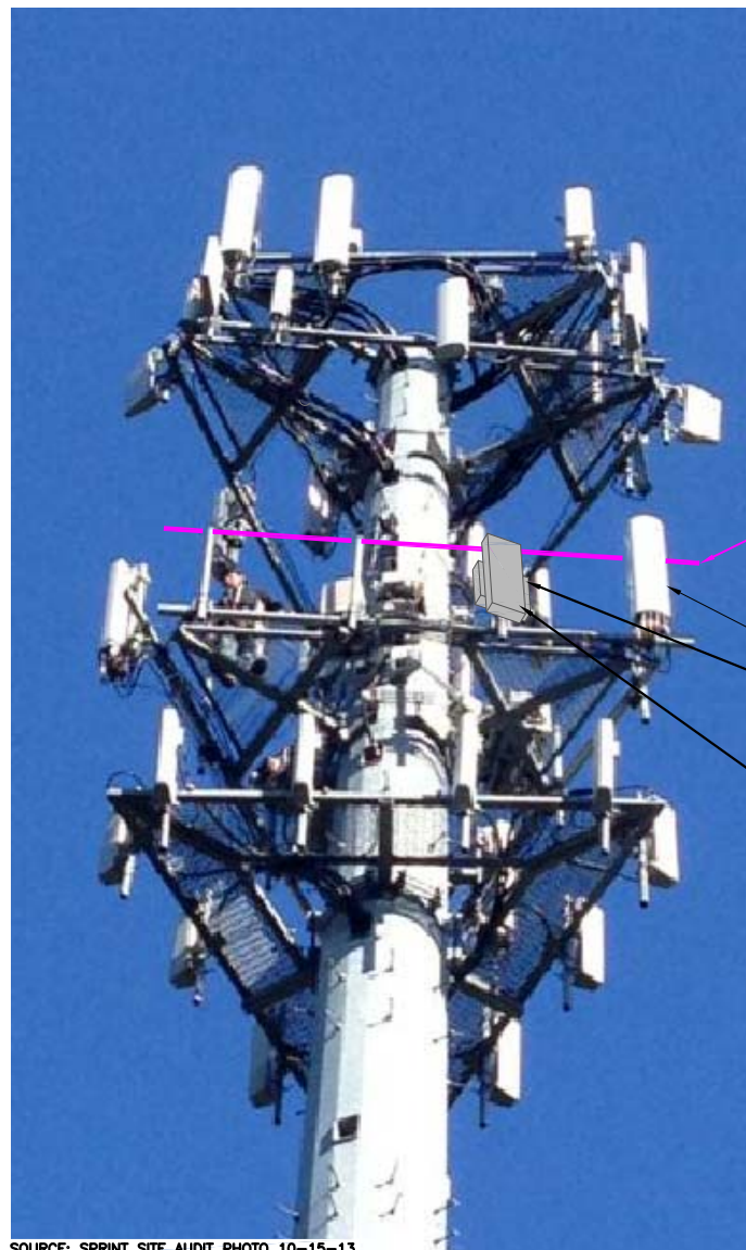
SOURCE: SPRINT SITE AUDIT PHOTO 10-15-13 2.5 ANTENNA AND RRH PHOTO DETAIL AND EQUIPMENT SCHEMATIC SCALE: N.T.S.
