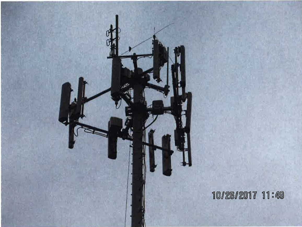
Photo 1: Photo illustrating the monopole with Appurtenances shown.
