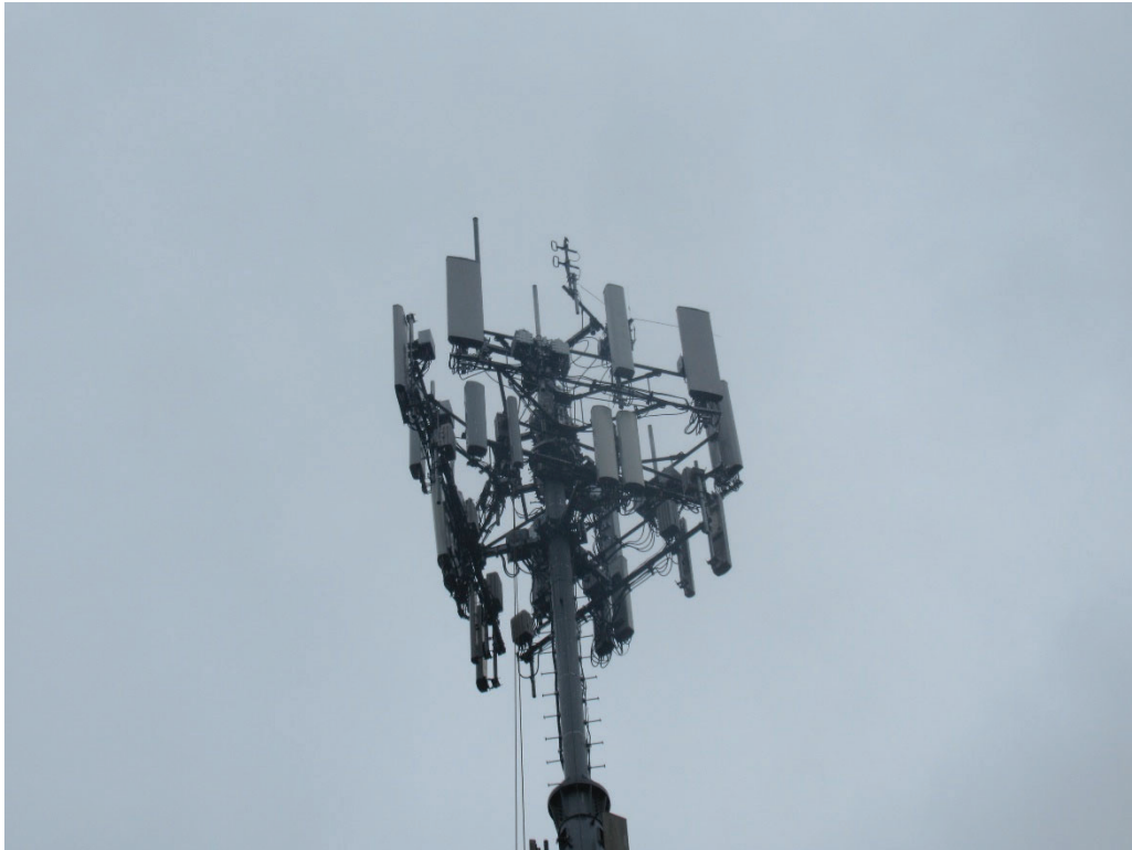
Photo 1: Photo illustrating the Tower with Appurtenances shown.
